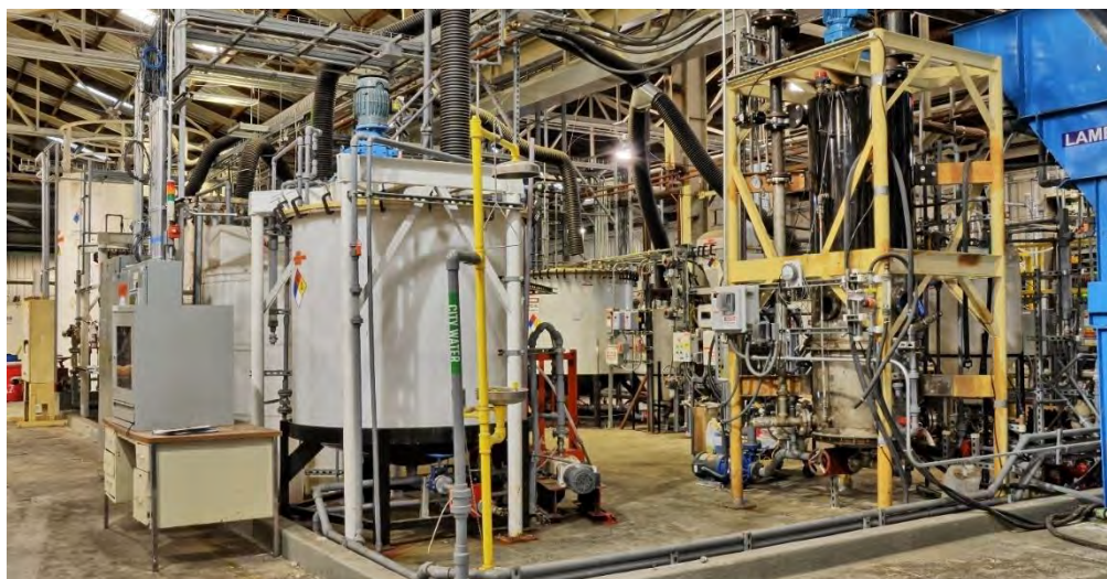
Figure 2. CaCO 3 cement pilot plant.
